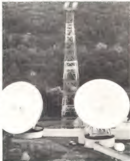
AT & T satellite dishes and microwave tower
